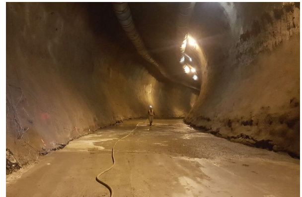
Excavations of the diversion tunnels are substantially completed. They will be temporarily coated with shotcrete until the permanent concrete liner is installed.
