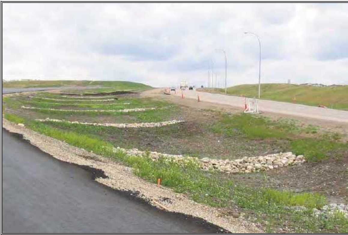
A system of well-installed rock check dams (properly spaced and extended up the sides of the channel) on a road construction project.
