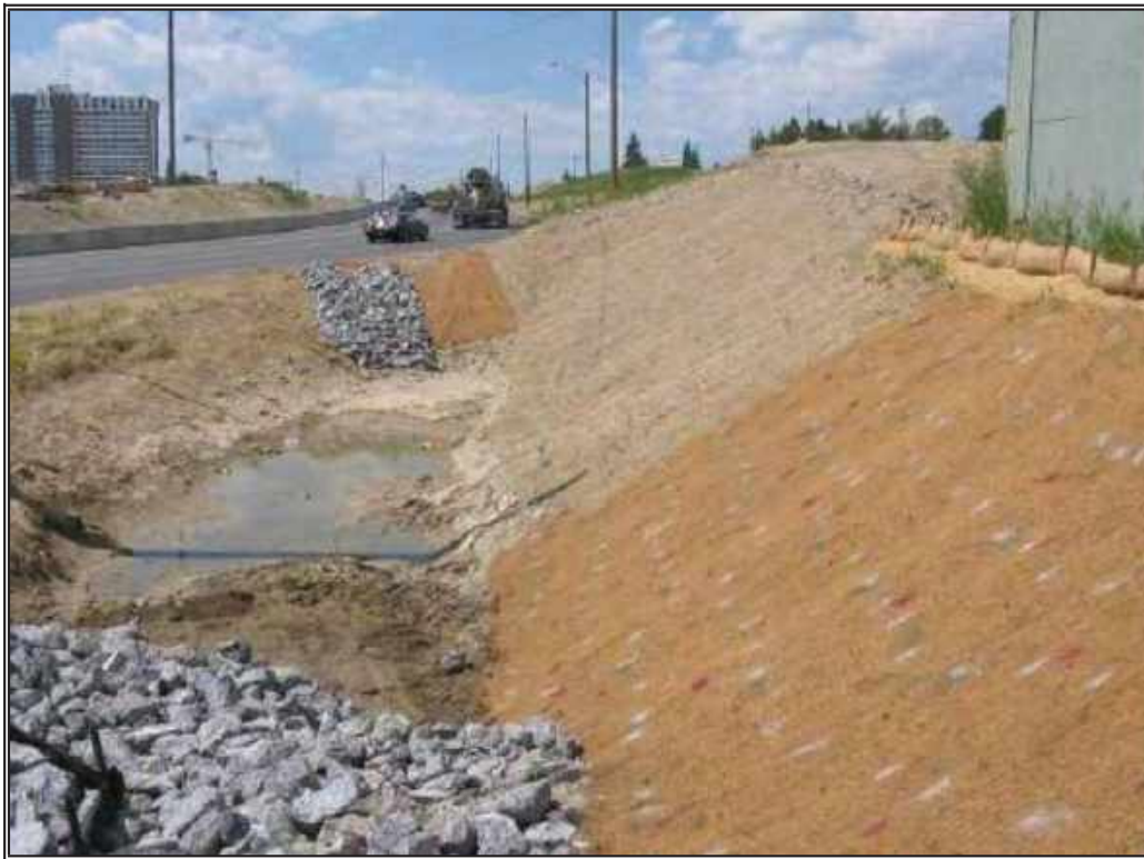
Simple sediment trap, with stabilized inlet and outlet and application of an erosion control blanket to protect side slopes.
