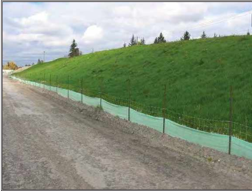
Photo 9: Providing vegetation cover on this soil stockpile controls erosion and helps preserve the biological, chemical and physical integrity of the soil. Perimeter control (silt fence) was installed around the pile to control migration of sediment during stabilization.
