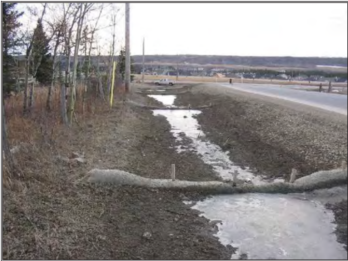
Straw wattles provide an excellent type of ditch check in small ditches conveying small volumes of run-off.
