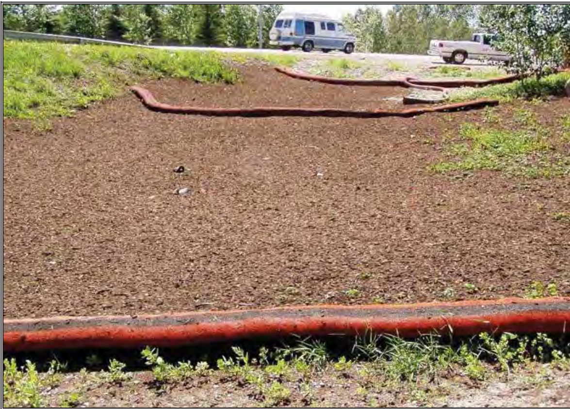
Photo 21: Combination of compost socks and a compost blanket applied to control erosion adjacent to a sensitive creek. A design seed mix was incorporated with the application, resulting in long-term erosion control. Biodegradable compost sock liners are also available.
