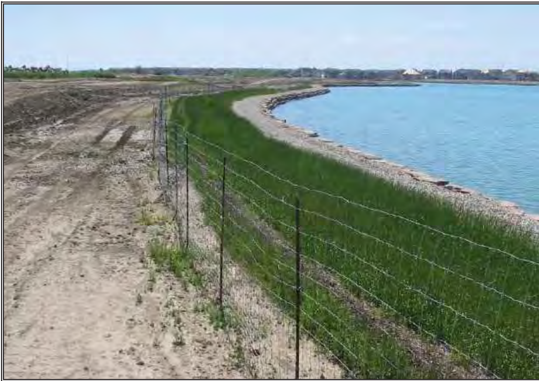
Protection of water body adjacent to a stripped area of land is enhanced with a seeded compost berm and compost blanket (promotes filtering of sediment-laden run-off and provides an erosion-resistant buffer.
