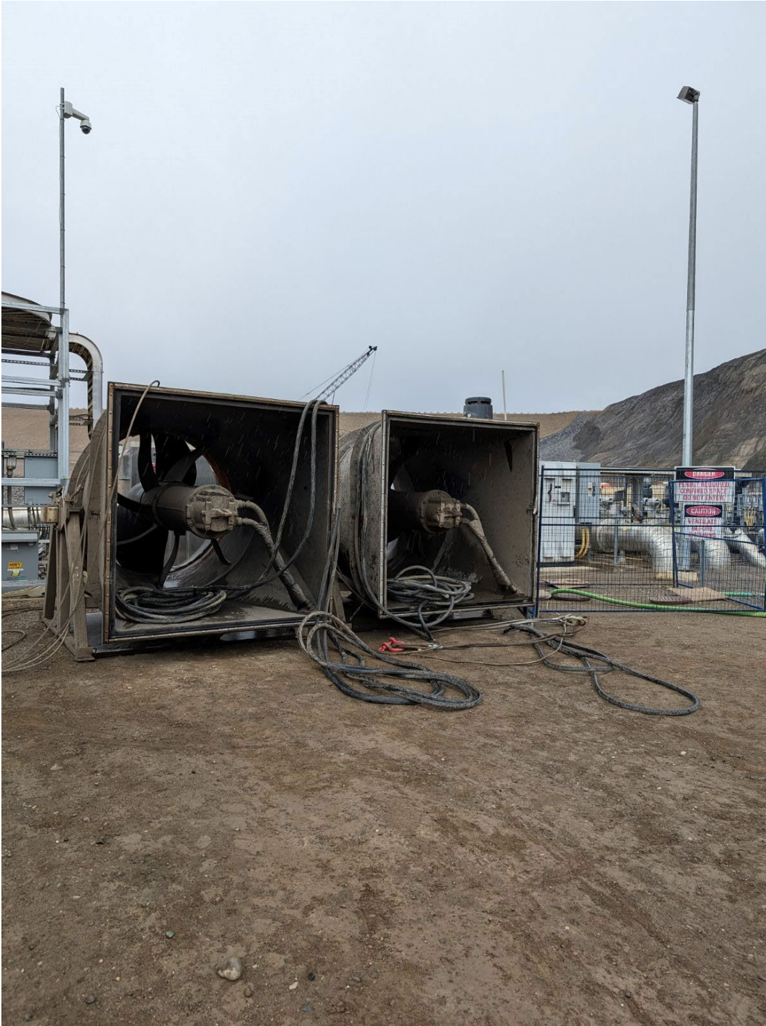
Photo 2. Horizontal propeller pumps – which provide the attraction flows at the temporary facility – were pulled from the pump station for inspection and repair (April 15, 2024).
