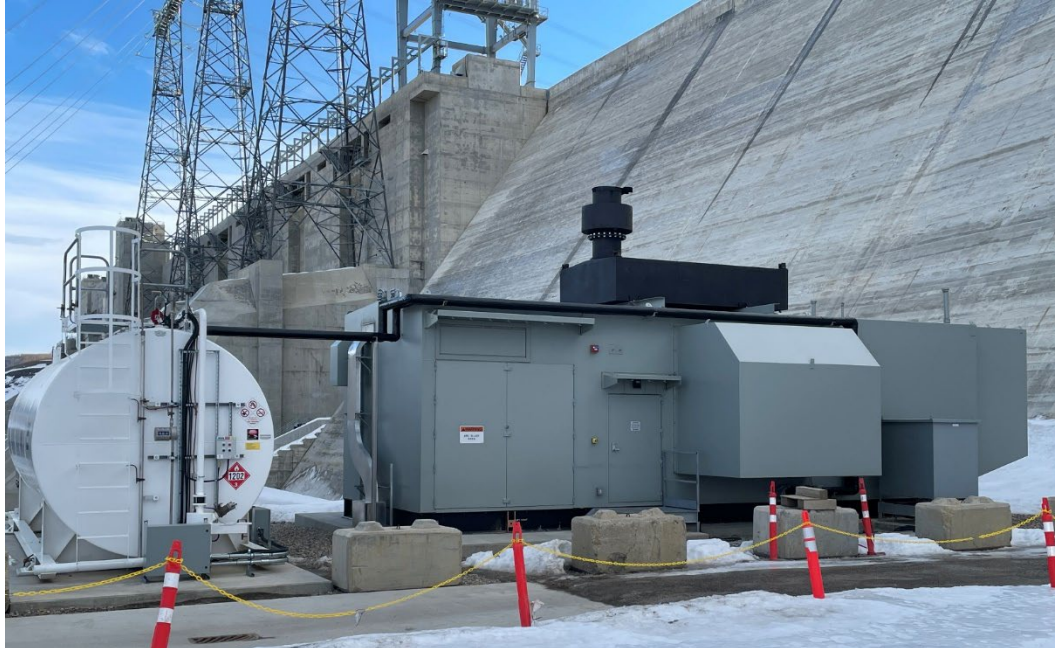
Figure A-24 Powerhouse Diesel Generator (January 2026)
