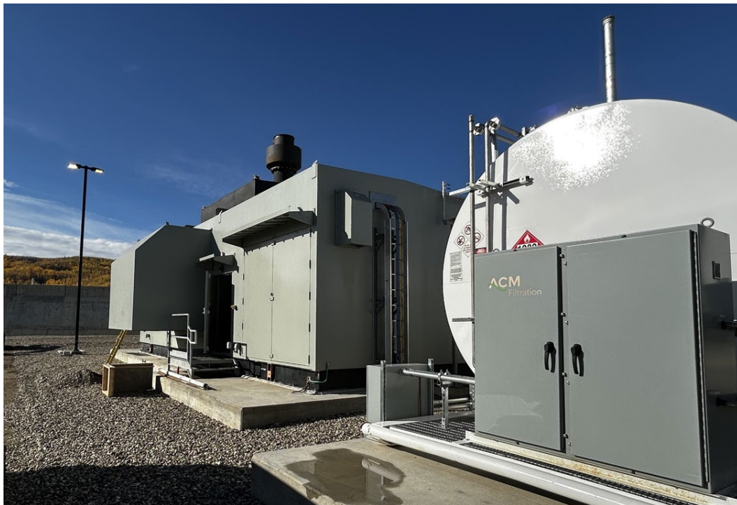
Figure A-25 Spillway Diesel Generator (January 2026)
