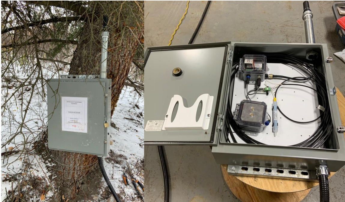
Figure 6: An example of a weather-resistant cabinet at a shore-based TDG station (left inset; Stn_112.5L) deployed as part of the Site C TDG Monitoring Array, 2023. The interior of the cabinet and the components housed within the cabinet are shown in the right inset.
