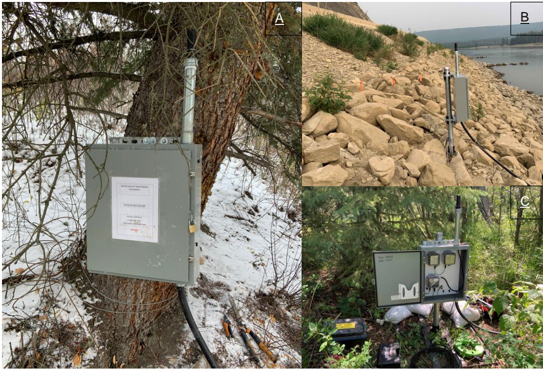
Figure 6: An example of deployment of a weather-resistant cabinet at a shore-based TDG station using lag bolt to secure the cabinet to a tree (inset A; Stn_112.5L). The cabinets were also deployed by mounting them to a steel pole with the base secured to either a rock (inset B; Stn_107.1L) or onto a steel frame (inset C; Stn_134.1R). The components of a shore-based station housed within the cabinet are shown in inset C.
