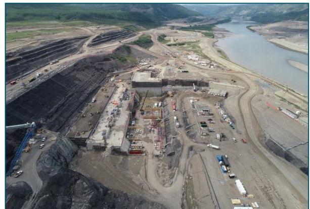
The work on the south bank is in close proximity to the Peace River
