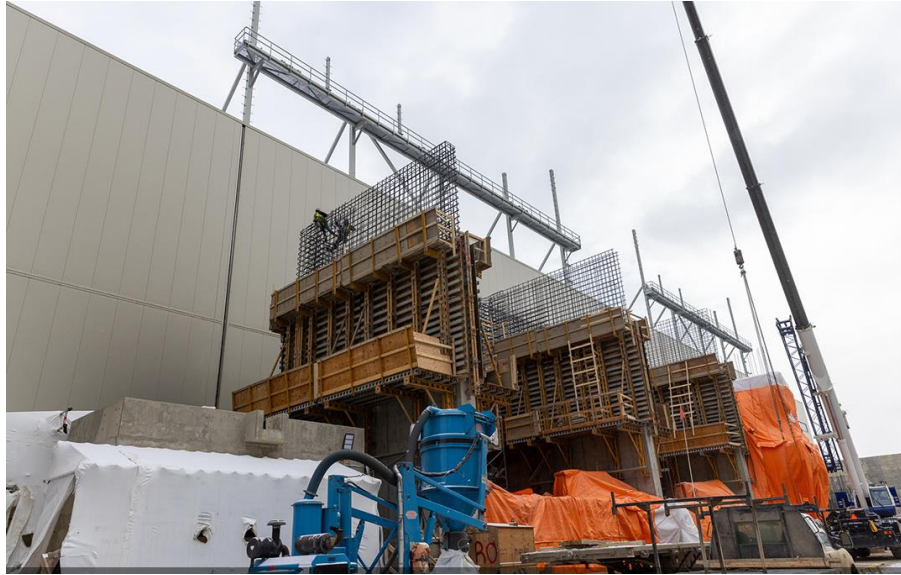
Figure A-8 Rebar framing is installed for the second of three transformer pads and blast walls. These walls are designed to contain fire and protect neighbouring units | March 2024
