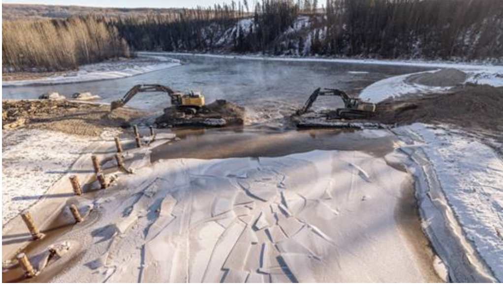
Figure A-1 Removal of a causeway that was blocking a section of river channel during the construction of fish habitat. Water from the river will gradually fill the channel | January 2024
