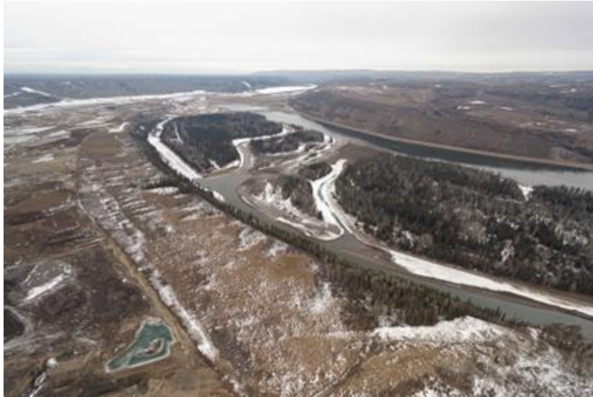
Figure A-3 The newly opened fish habitat located downstream of the earthfill dam. Construction on the fish habitat included deepening the channels and embedding logs in the channels for fish to rest | February 2024
