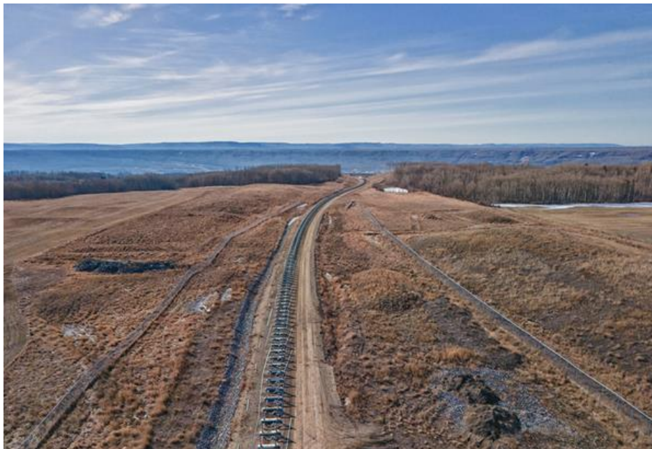
Figure A-9 The removal of the conveyor (transported glacial till for the core of the earthfill dam) framework from the south portion of the five-kilometre-long conveyor right-of-way is scheduled to be complete by late summer | March 2024
