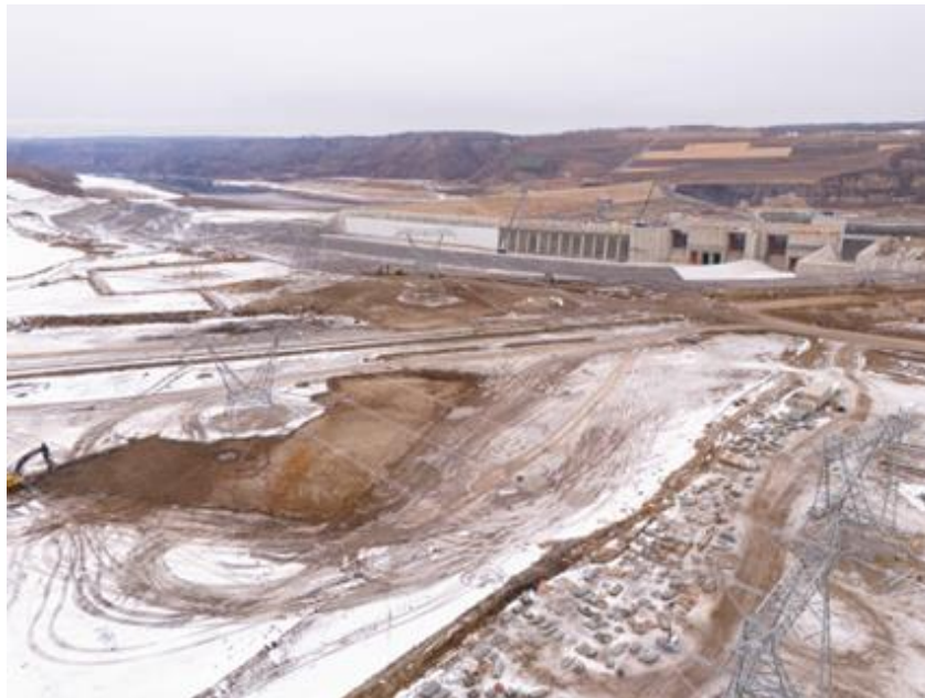
Figure A-4 Three one kilometre long, 500 kilovolt transmission lines will connect the Site C substation to the Site C powerhouse | February 2024
