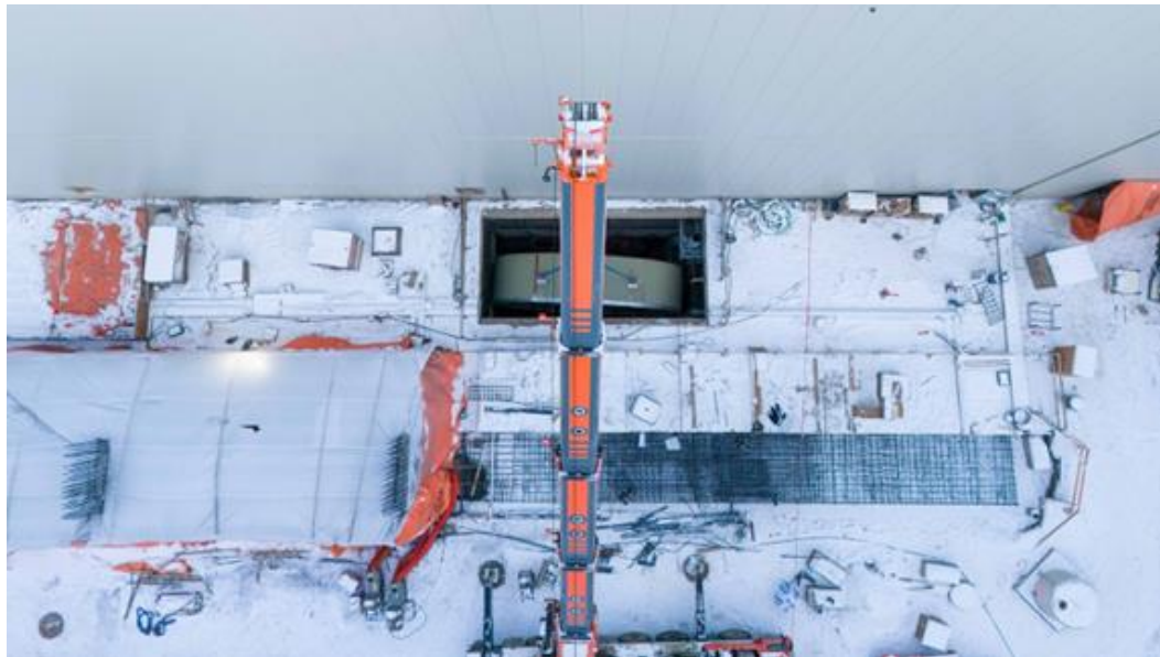
Figure A-2 The lower flexible coupling (located between the bottom of the penstock and the turbine scroll case) is lowered through the unit 6 access hatch at the coupling chamber | January 2024
