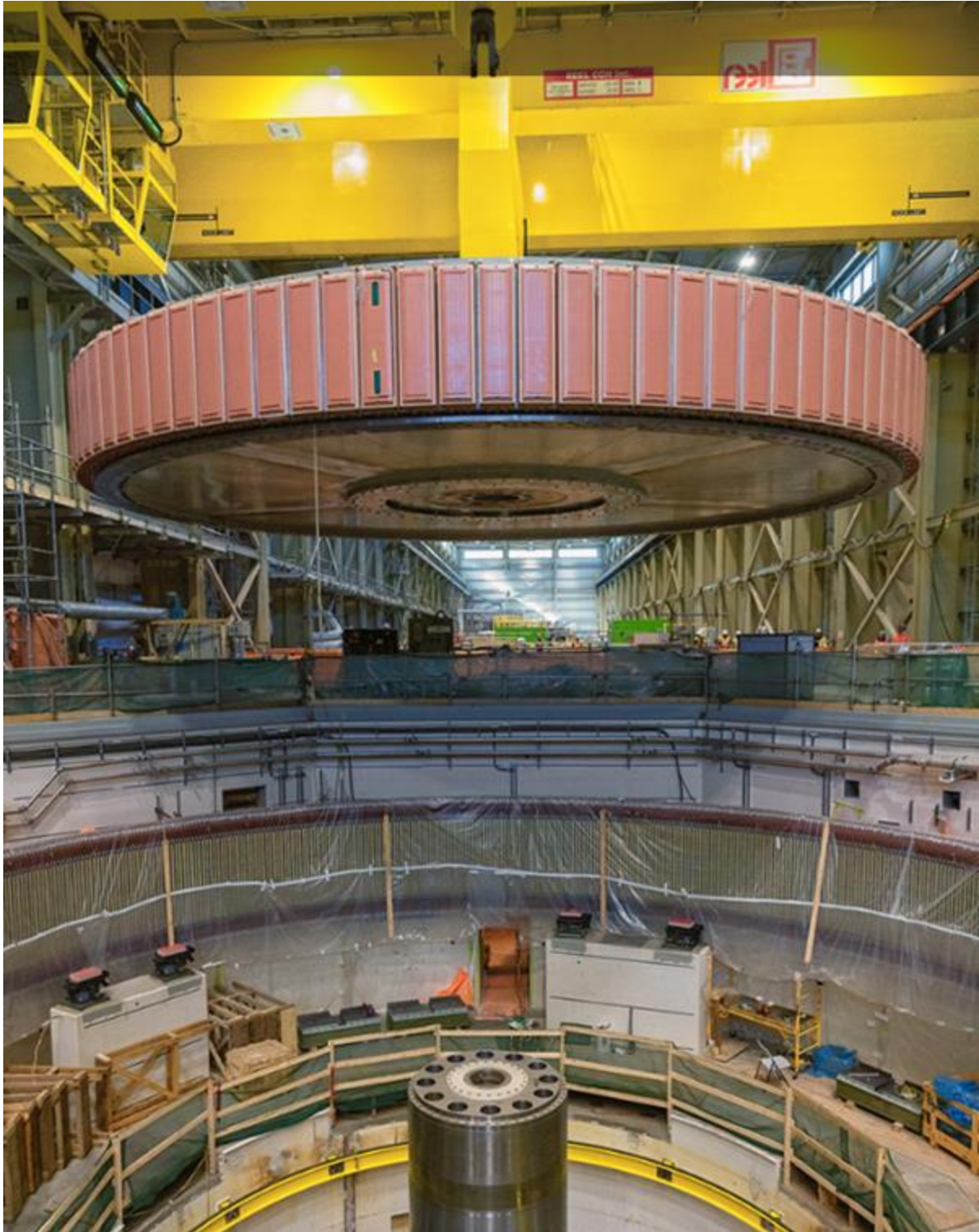
Figure A-7 The unit 3 rotor (part of the generator) is lowered into position | March 2024
