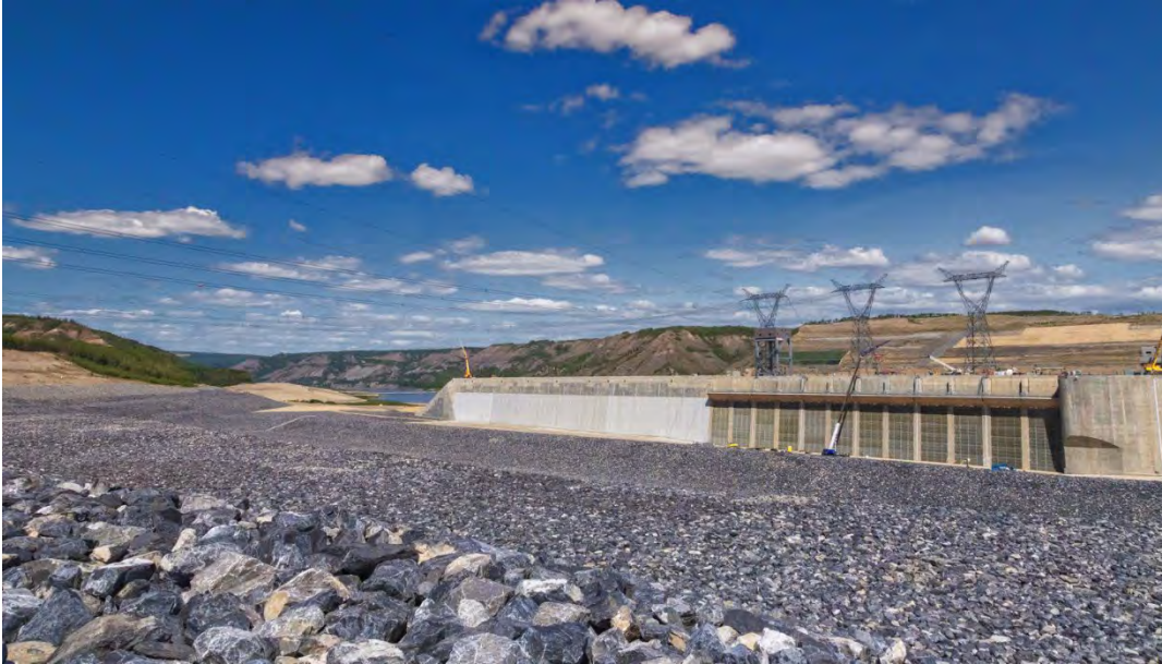
The transmission towers at the Site C dam are connected to the Southbank substation, with lines strung over the approach channel. See more construction photos in our gallery.
