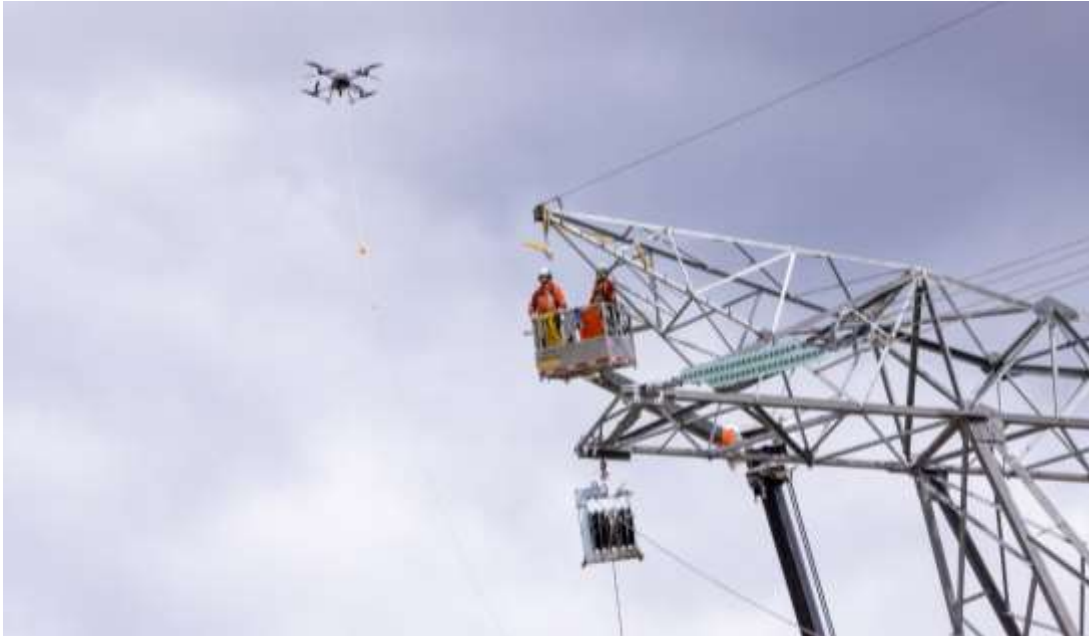
A drone is used to string the transmission lines from the substation to the powerhouse. See more construction photos in our gallery.
