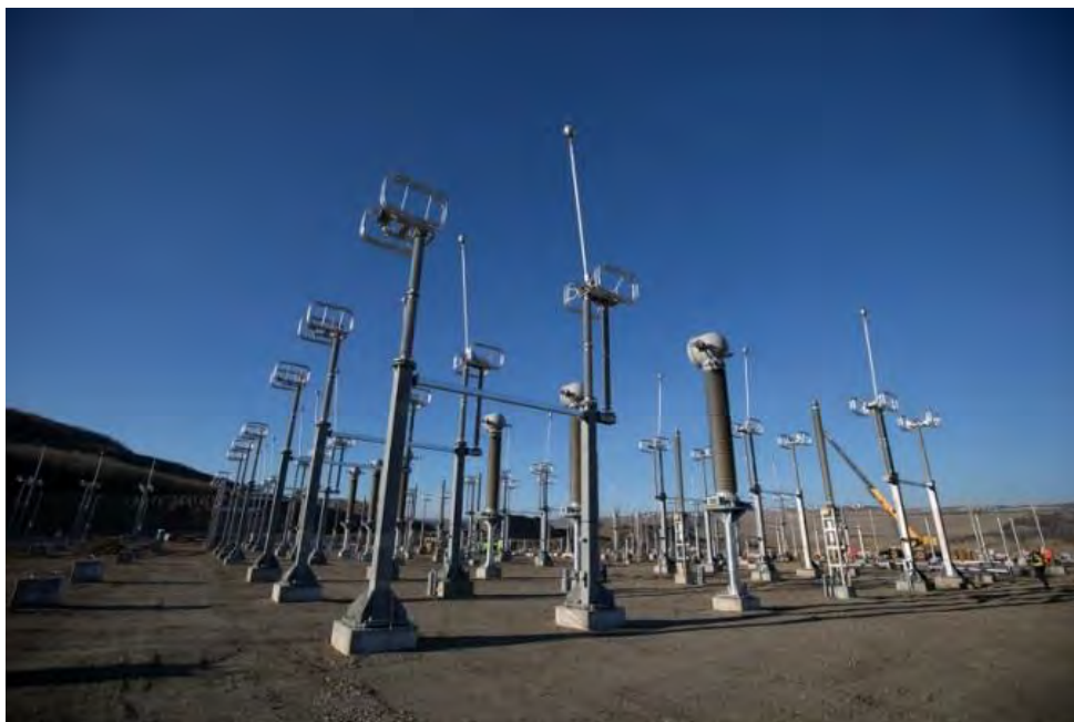
Figure A-30 500kV Electrical Equipment at the Site C Substation (October 2018)
