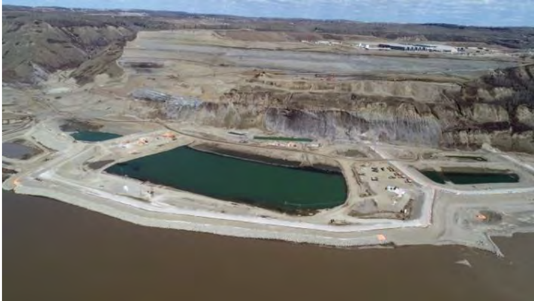
Figure A-13 Left Bank Inlet Portal Cofferdam and Outlet Portal Cofferdam (May 2018)
