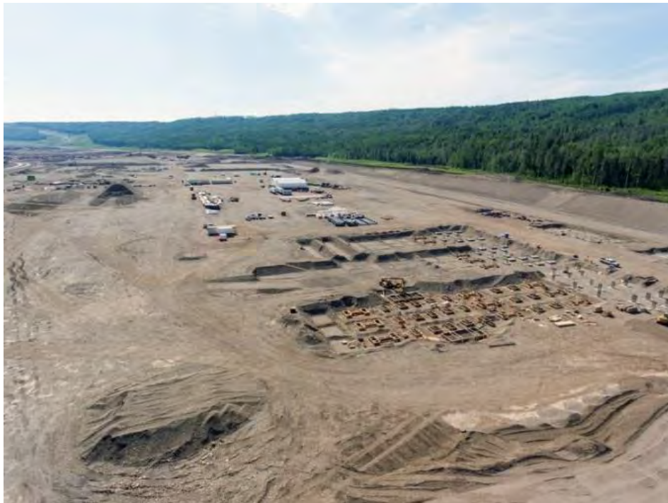
Figure A-16 Installing Concrete Forms for the Substation on the Right Bank (June 2018)
