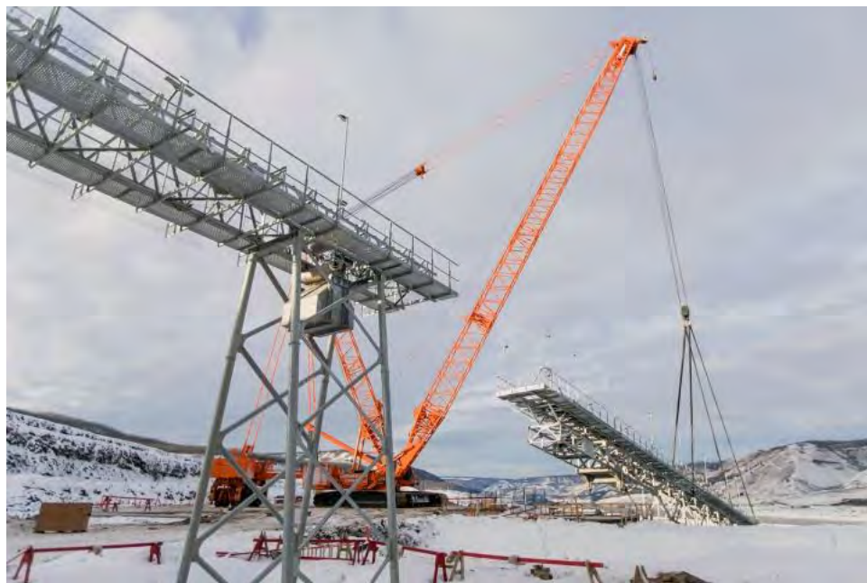
Figure A-2 Installing Conveyor Equipment at the Approach Channel and Powerhouse Buttress on the Right Bank (January 2018)
