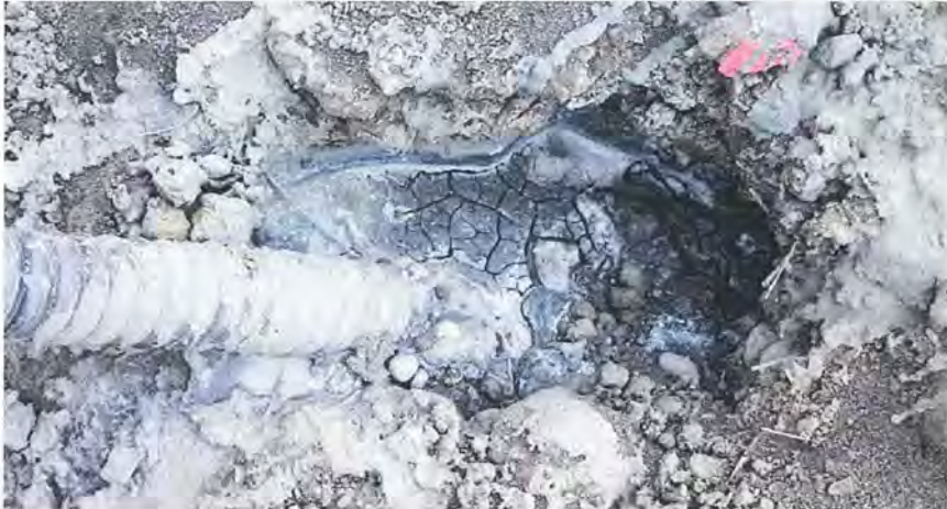
Severely shrinking grout at rock dowel in soil nail slopes
