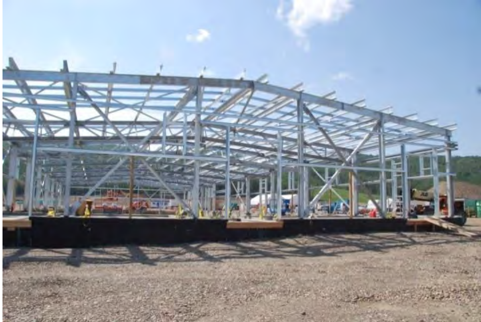
Figure A-19 Substation Control Building Steel Structure on the Right Bank (August 2018)
