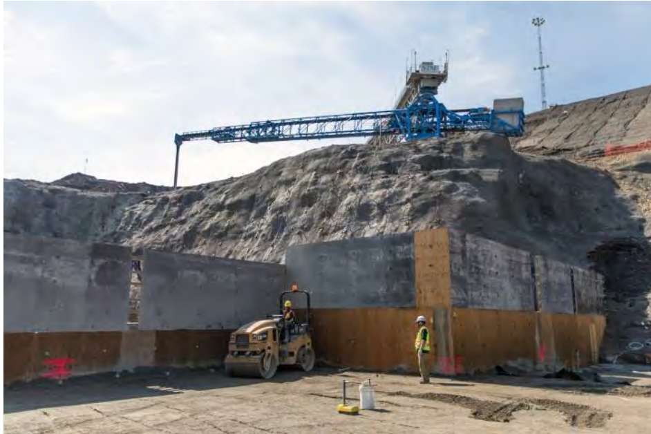
Figure A-15 Roller-Compacted Concrete Placement and Shotcrete Application for the Spillway Buttress on the Right Bank (June 2018)
