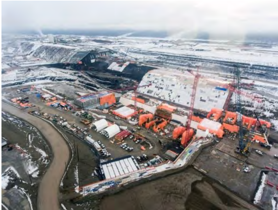
Figure A-33 Construction of the Earthfill Dam on the Left Bank (November 2018) Roller-Compacted Concrete Buttress on the Right Bank, with the Concrete Insulated for Winter (November 2018)
