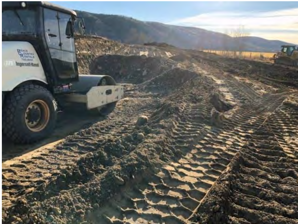
Figure A-28 Start of Highway Realignment Work at Cache Creek West (October 2018)
