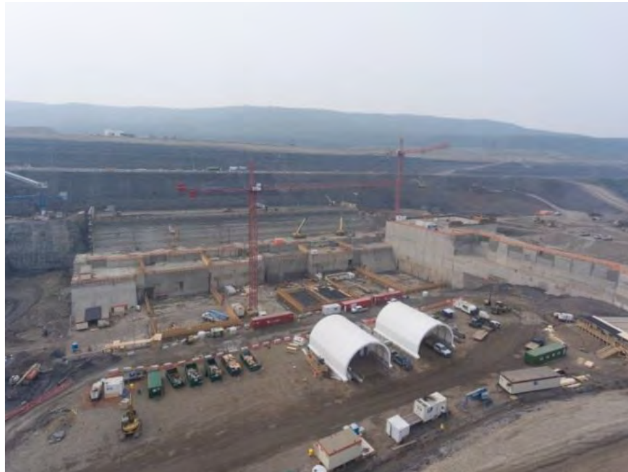
Figure A-22 Powerhouse Buttress and Generating Station and Spillways Civil Works Laydown Area (August 2018)
