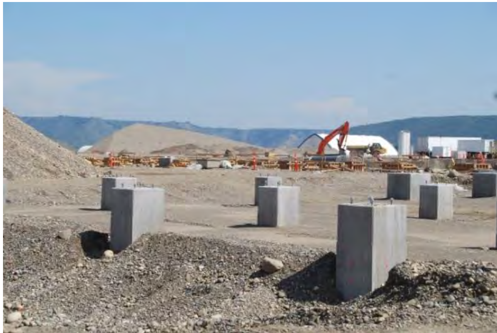
Figure A-20 Concrete Pedestals and Concrete being Placed in Forms for the Substation (August 2018)
