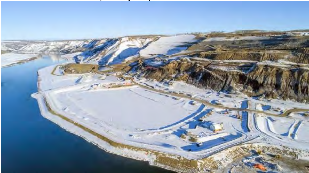
Figure A-4 Aerial View of the Left Bank with Cofferdam and Excavation, Facing Northwest (February 2018)
