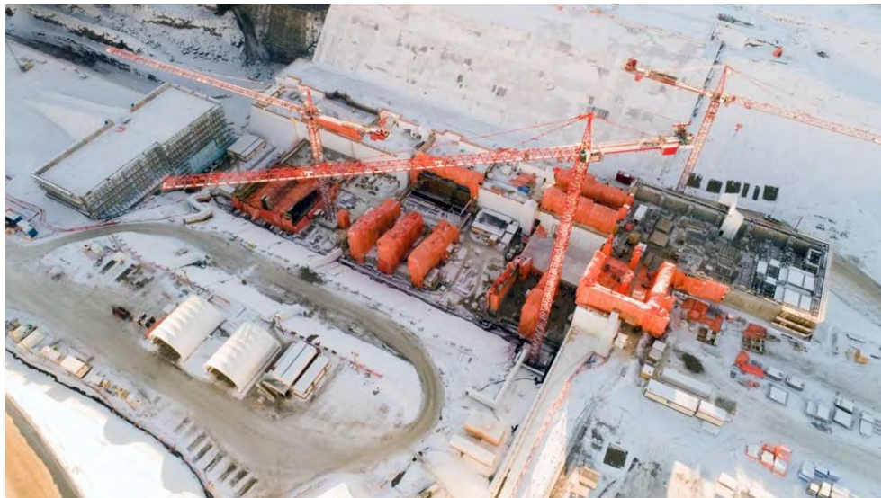
Figure A-34 Powerhouse and Main Service Bay on the South Bank (December 2018)
