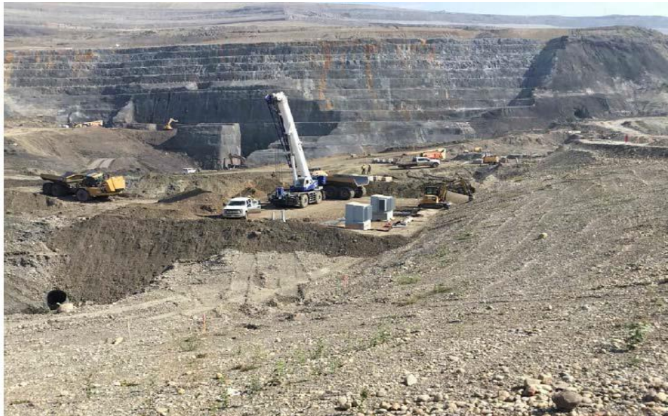
Figure A-4 Inlet Cofferdam Facing North; Crane Placing Transformers for the Diversion Tunnel Operations. Photo taken August 2018.
