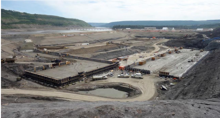
Figure A-3 Overview of the Powerhouse Buttness, Service Bay Pad, Tailrace Wall, and Generating Station & Spillways Laydown Areas. Photo taken July 5, 2018.
