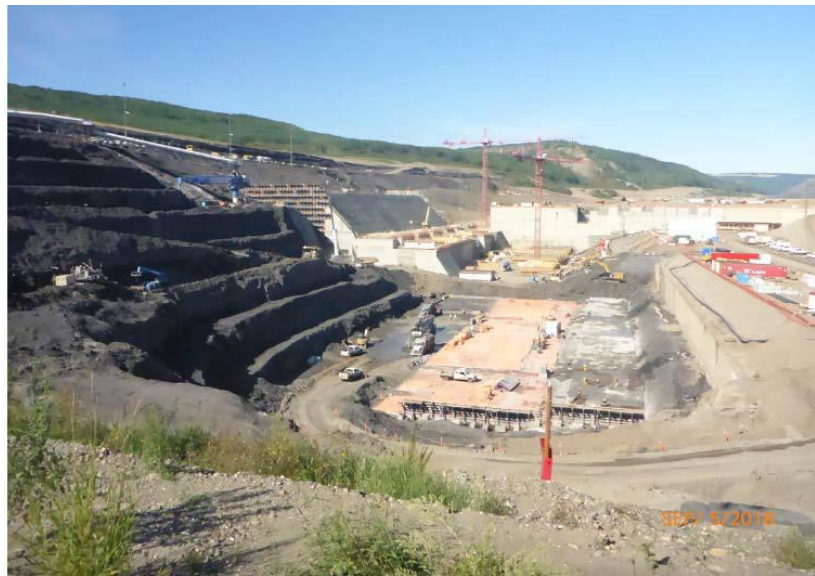
Figure A-8 Hydrovac Trucks Supporting Foundation Preparation for the Spillway Buttress Apron. Photo taken September 5, 2018.
