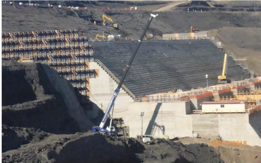
Figure A-9 Removal of Formwork from the East Face of the Powerhouse Buttress. Photo taken September 5, 2018.
