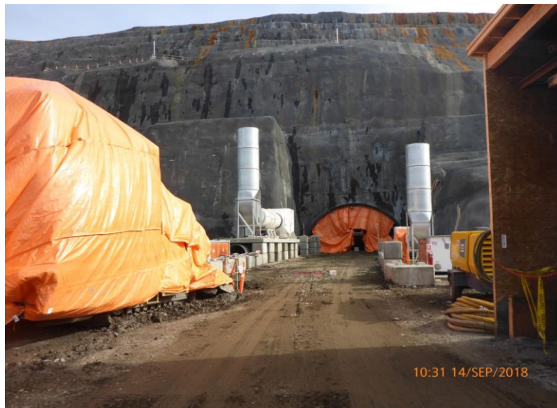
Figure A-10 Road Header and Tunnel Entrance Hoarded; Dust Suppression System Raised. Photo taken September 14, 2018.
