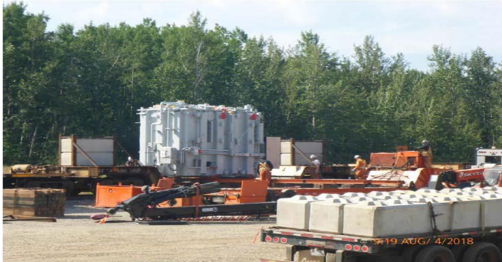
Figure A-5 Transformers Being Winched onto Flat Deck for Deliver to the Substation. Photo taken August 4, 2018.
