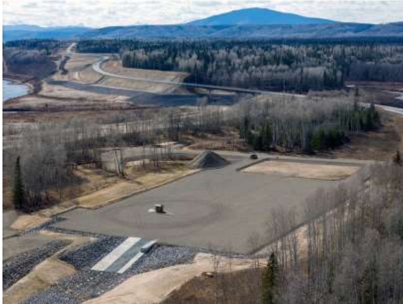
Figure A-2 The new Lynx Creek boat launch is being built just off the realigned Highway 29 near the Lynx Creek bridge. The boat launch will access the future Site C reservoir | April 2024
