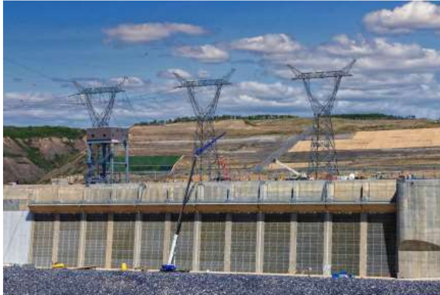
Figure A-4 The second of three transmission towers was installed in April. Conductor stringing was completed in early May to connect these three towers to the Site C substation | May 2024
