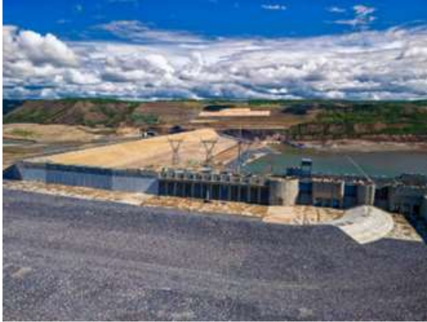
Figure A-10 The upstream side of the Site C generating station where water will flow from the approach channel through the intake gates to the generating units, or into the spillways | June 2024
