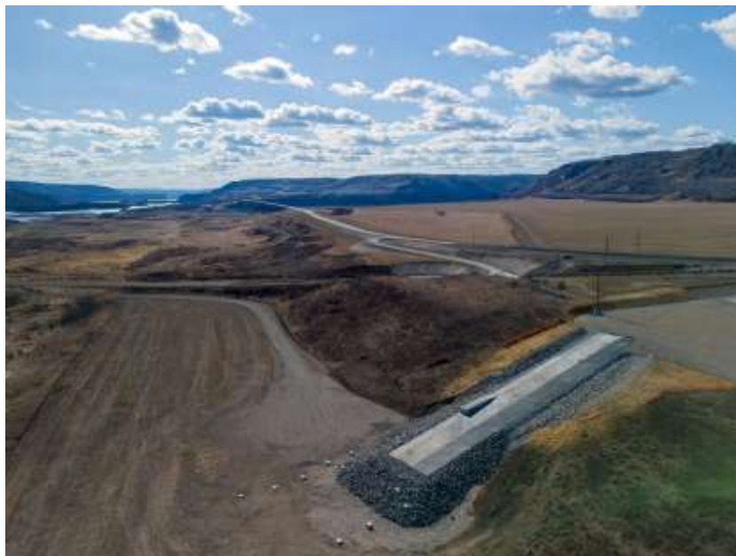
Figure A-3 The new Halfway River boat launch near the east-end of the Halfway River Bridge. The boat launch will access the future Site C reservoir | April 2024
