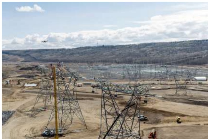
Figure A-7 Stringing of the conductor for one of the transmission lines connecting the Site C substation to the powerhouse. A drone is used instead of a helicopter to lift the pulling line. This pulling line is connected to the transmission line conductor to string the conductor onto the transmission towers | May 2024
