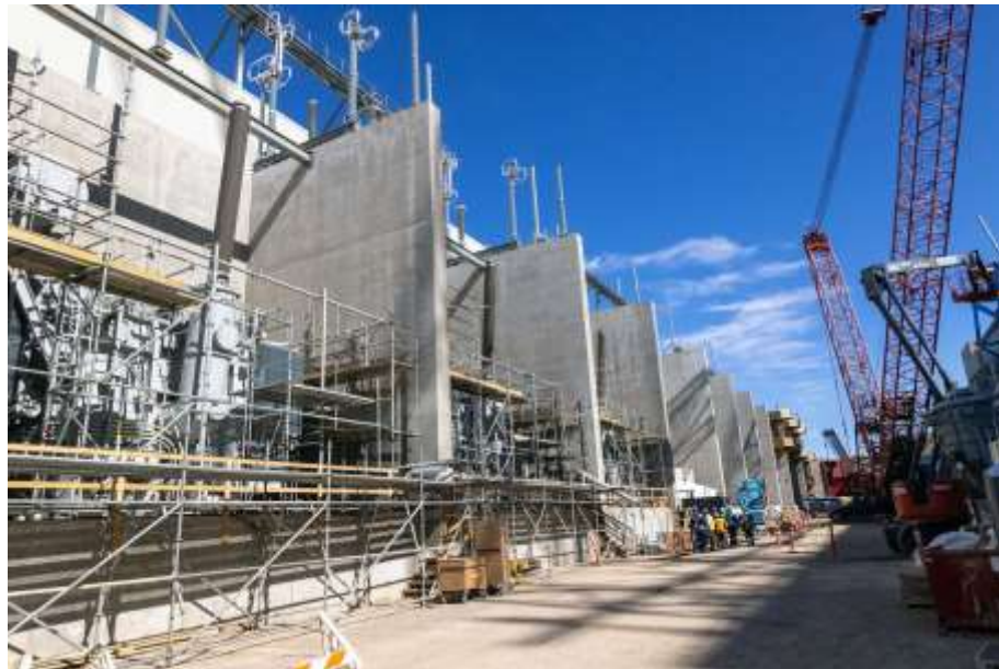
Figure A-5 The completed protection walls between the main transformers that step up the voltage from the generators from 13,700 volts to 500,000 volts. There are three sets of three protection walls that are now complete | May 2024
