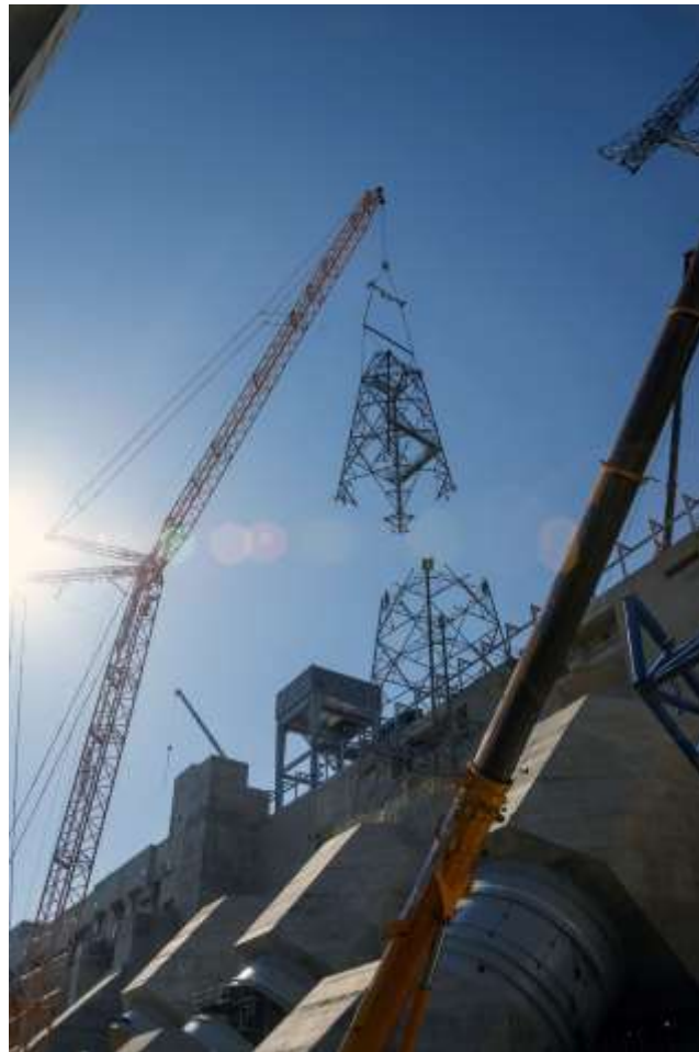
Figure A-1 A 440-tonne crane lifts the second section of the transmission tower into position on the intake structure. This tower is part of one of the transmission lines connecting the Site C substation to the powerhouse | April 2024
