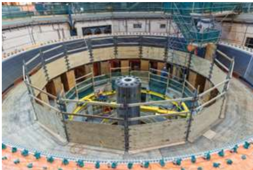
Figure A-9 Construction of generating unit 6. In the centre of the picture is the turbine shaft which connects the turbine to the generator rotor (once it is installed). The yellow lifting beam structure is used for ongoing maintenance | June 2024
