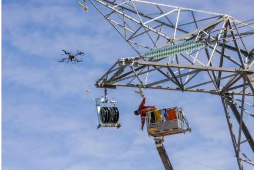
Figure A-6 Stringing of the conductor for one of the transmission lines connecting the Site C substation to the powerhouse. The drone lifts the pulling line while a powerline technician stands by to help guide the conductor through a sheave attached to the tower | May 2024
