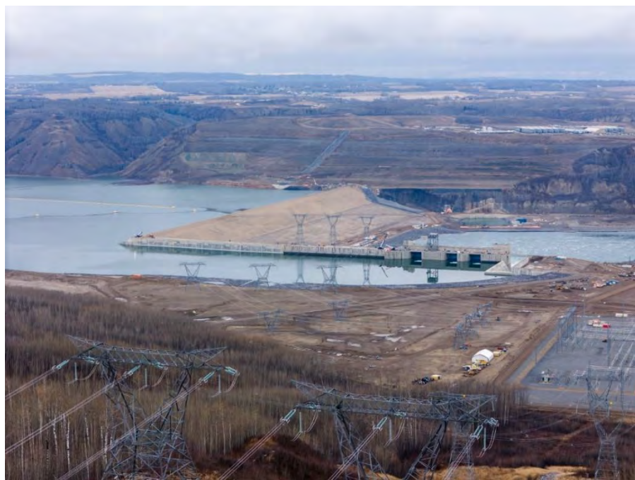
Figure A-11 Two 500-kilovolt transmission lines transport electricity generated at Site C into the BC Hydro transmission grid
