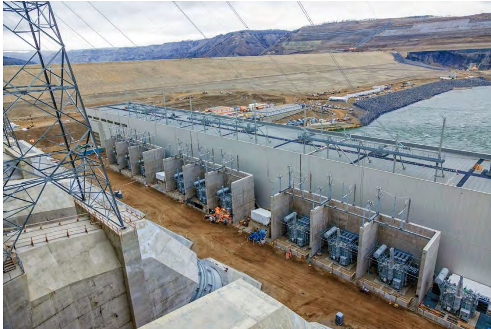
Figure A-3 Transmission connection is complete with all three sets of transformers connected
