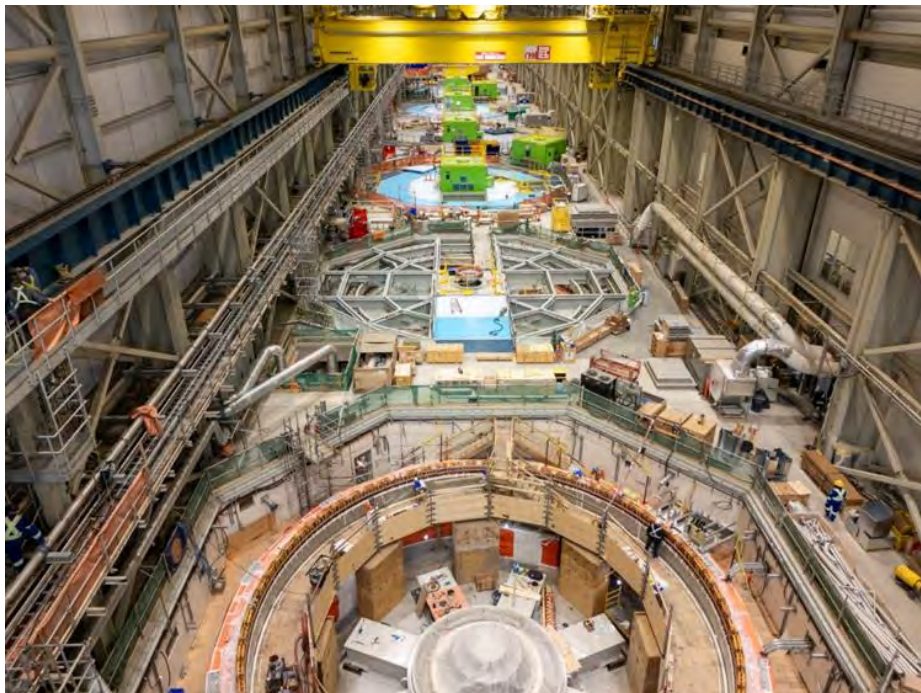
Figure A-9 Unit 6 through 1 in the powerhouse
