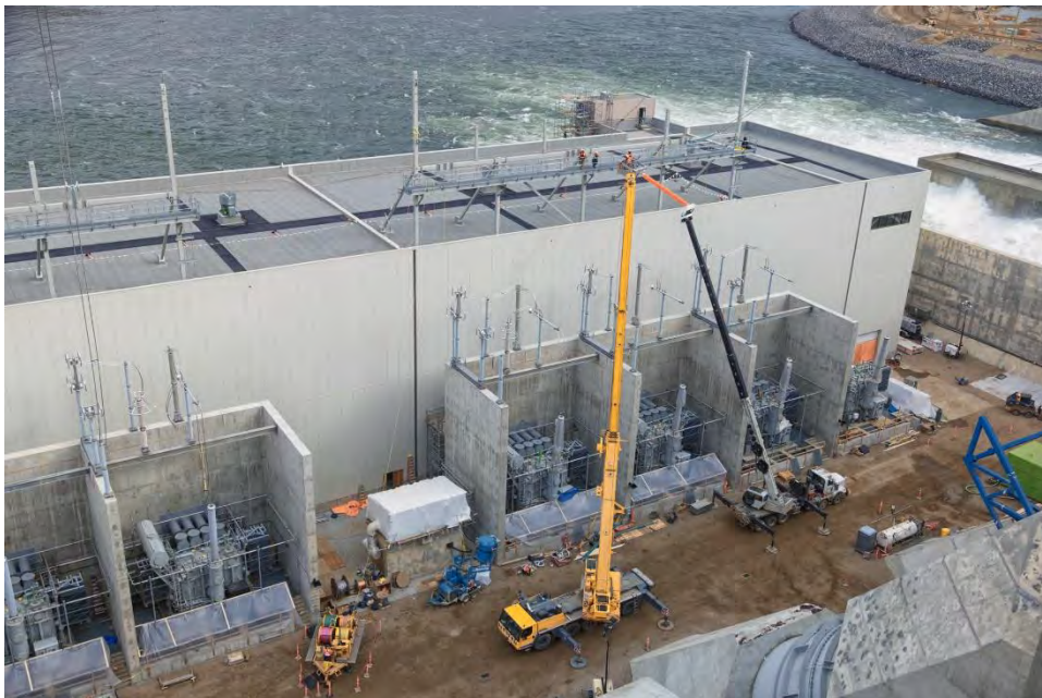
Figure A-2 The last set of three transformers is connected to the transmission system
