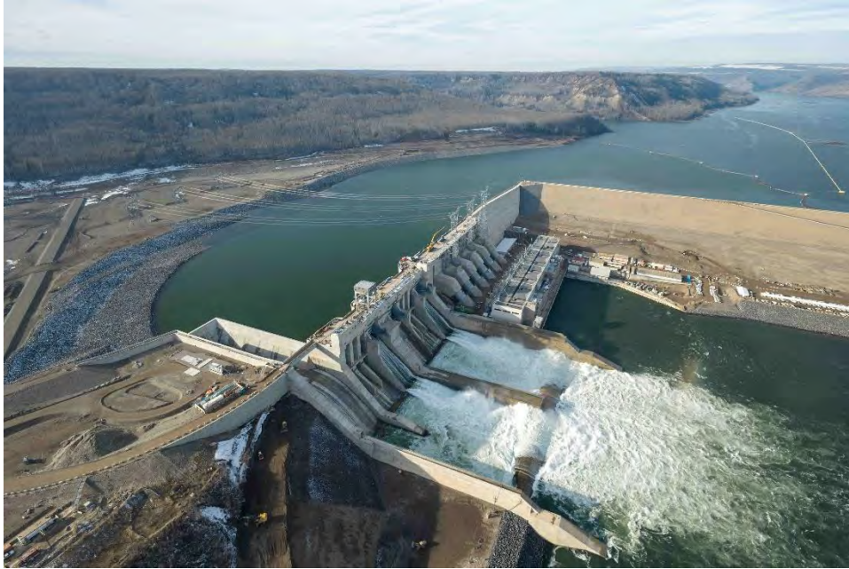
Figure A-12 Reservoir filling is underway with water flowing through the spillways to maintain downstream flows
