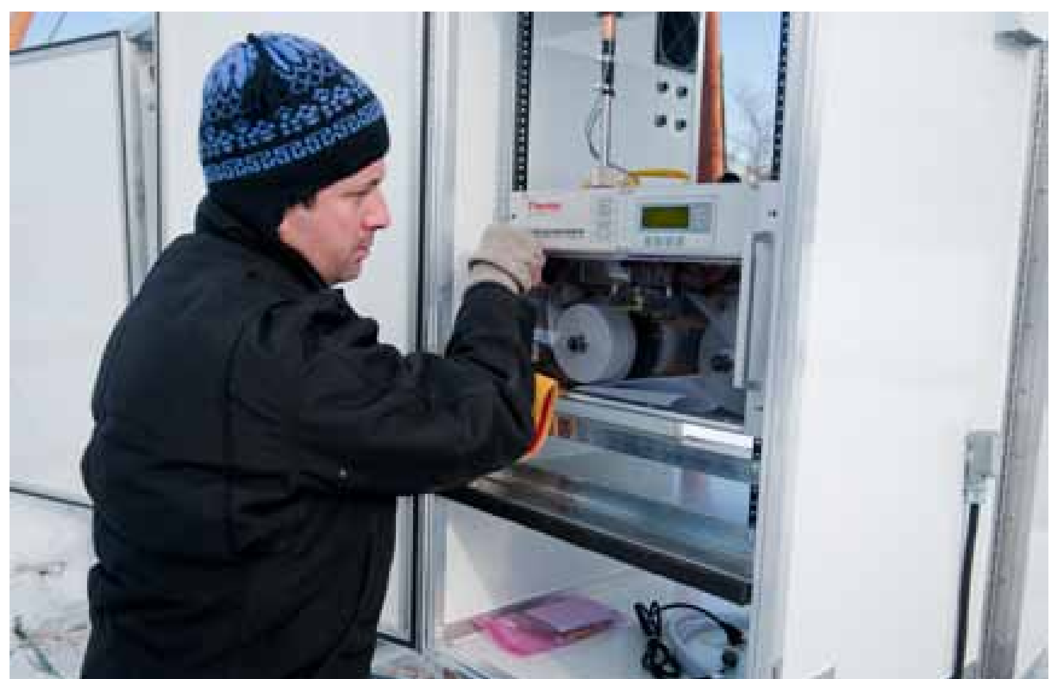
Installation of an air quality monitoring station at Old Fort
