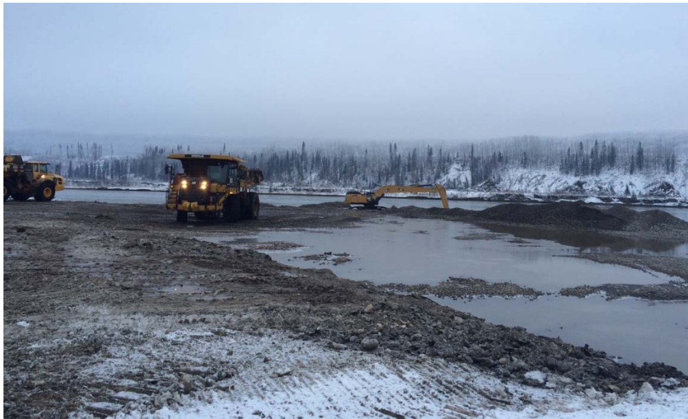
Figure 1. Temporary access platforms and haul-out areas used during in-river excavation of the bar referred to as Upper Site 109L.
