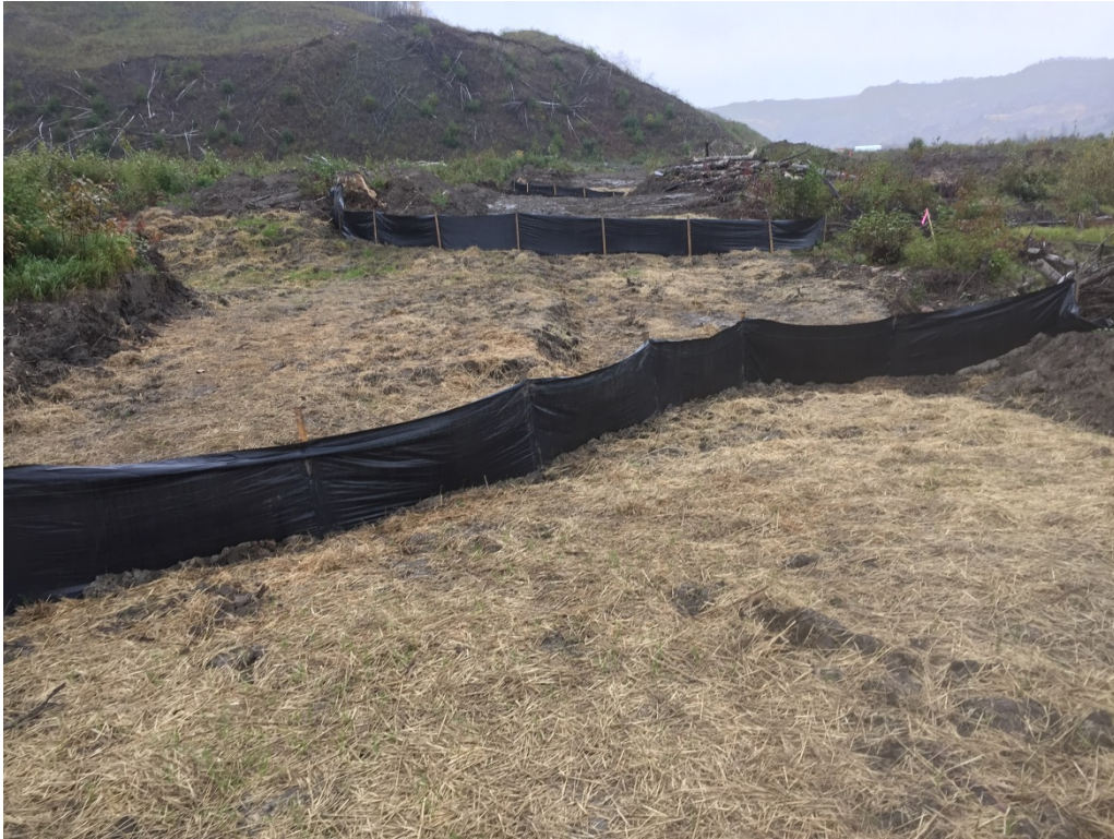
Figure 3. Example erosion and sediment control measures at an ephemeral channel in the area of construction of the causeway for the Moberly River construction bridge, Sept 30, 2016.
