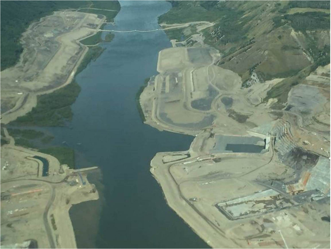
Aerial photo of the upstream cofferdam progress into the river (left), inlet cofferdam full of water (right), and upstream debris boom (top).
