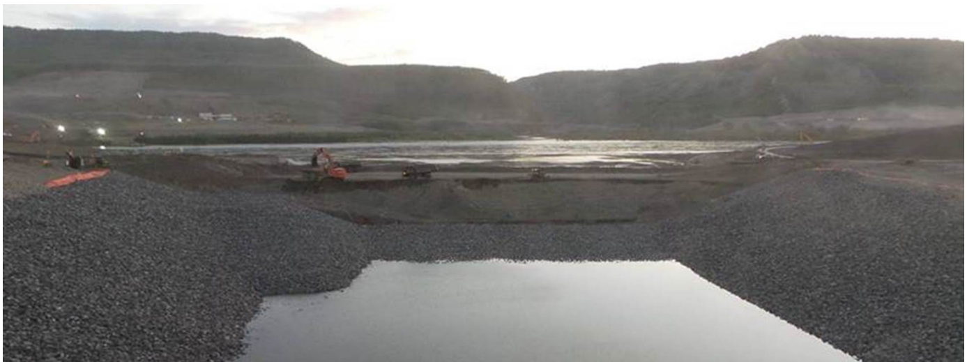
Top phase of the inlet cofferdam removed and an excavator beginning the next phase of cofferdam removal.
