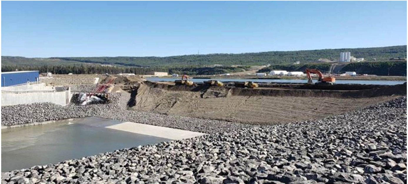
Water being pumped into the outlet cofferdam (left) while equipment removes material at the top of the outlet cofferdam.
