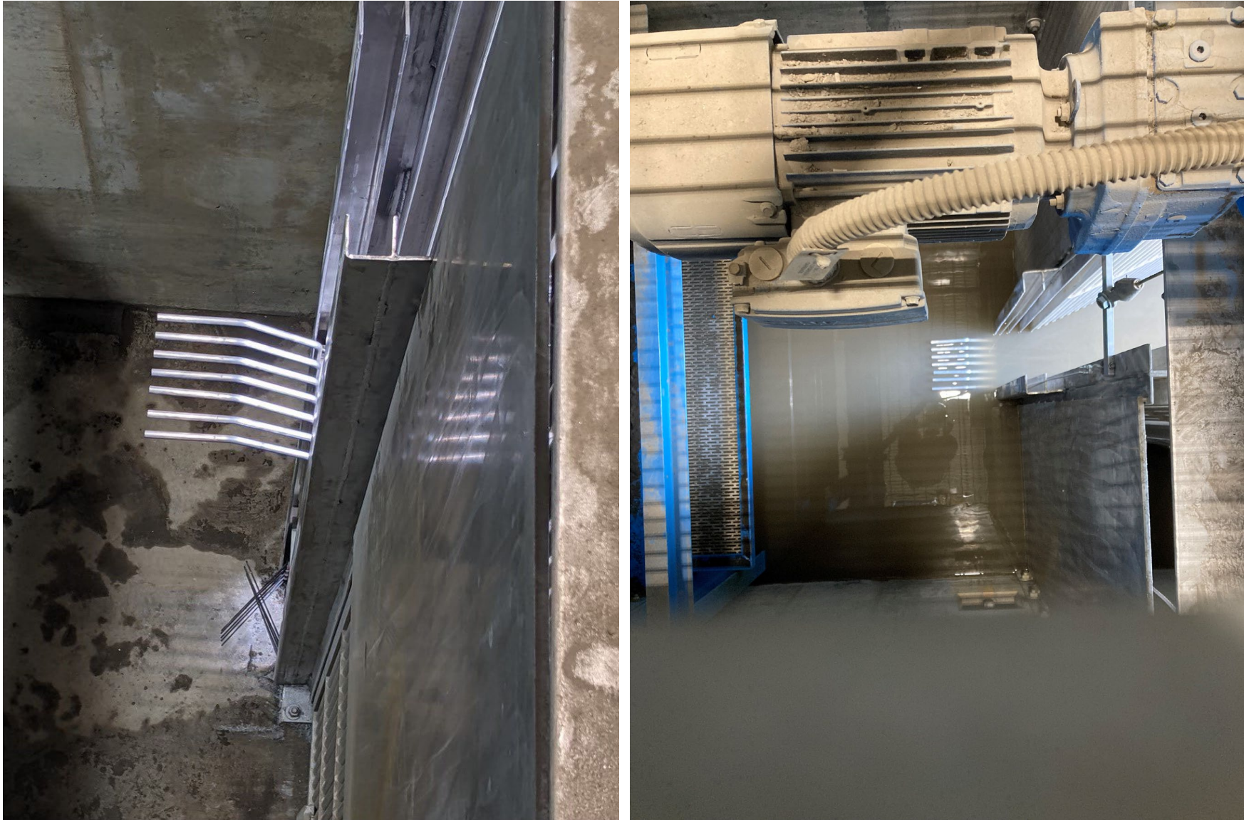
Photo 3. BC Hydro installed a finger weir and orifice panel in the vee-trap throat to improve trapping efficiency (left panel; June 9, 2022). Fish can now either swim over the finger weir or through the orifice and cod fingers to enter the pre-sort holding pool. BC Hydro set the finger weir at 23 cm below the water surface to match the existing hydraulic drop between fishway pools (right panel; June 13, 2022).
