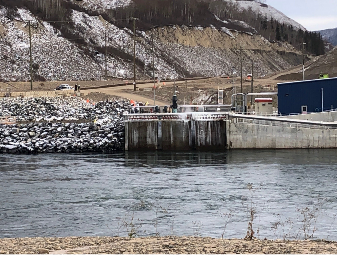
Photo 1. Cold air temperatures challenged the operation of the temporary facility during the reporting period (October 25, 2023).
