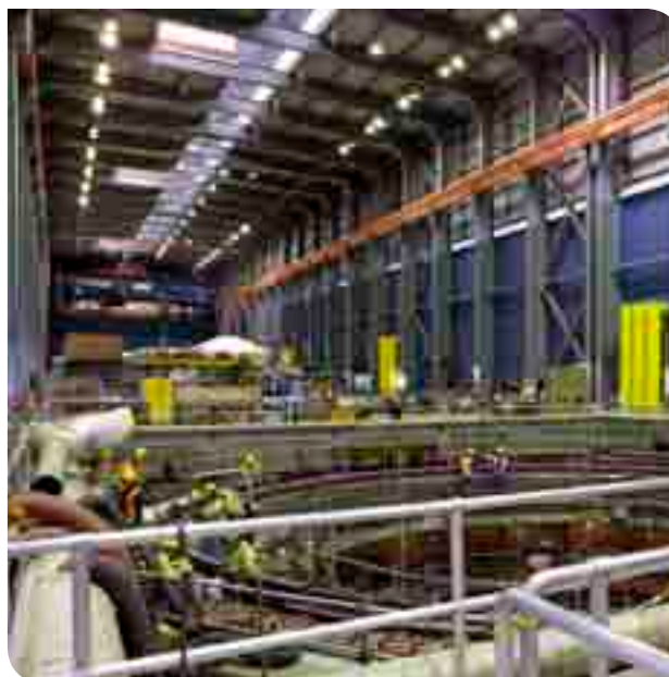
Maintenance and upgrading work on an electric generator at Peace Canyon generating station near Hudson's Hope (July 2009).
