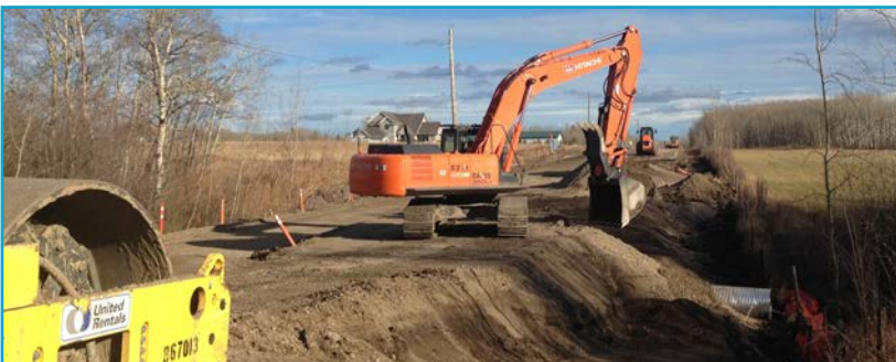
Ministry of Transportation and Infrastructure contractor A.L. Sims and Sons prepares 240 Road for paving.
