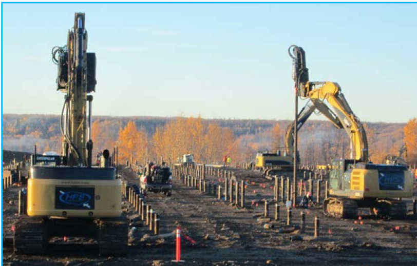
Excavators installing screw piles at the location of the worker accommodation camp.
