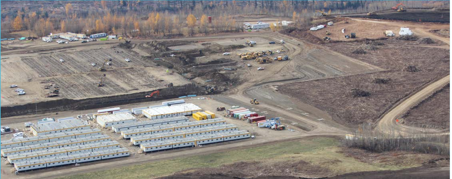
Aerial view of the north bank of the Site C dam site. A temporary 300-person modular complex houses ATCO workers as they build a 1,600-person worker accommodation facility.
