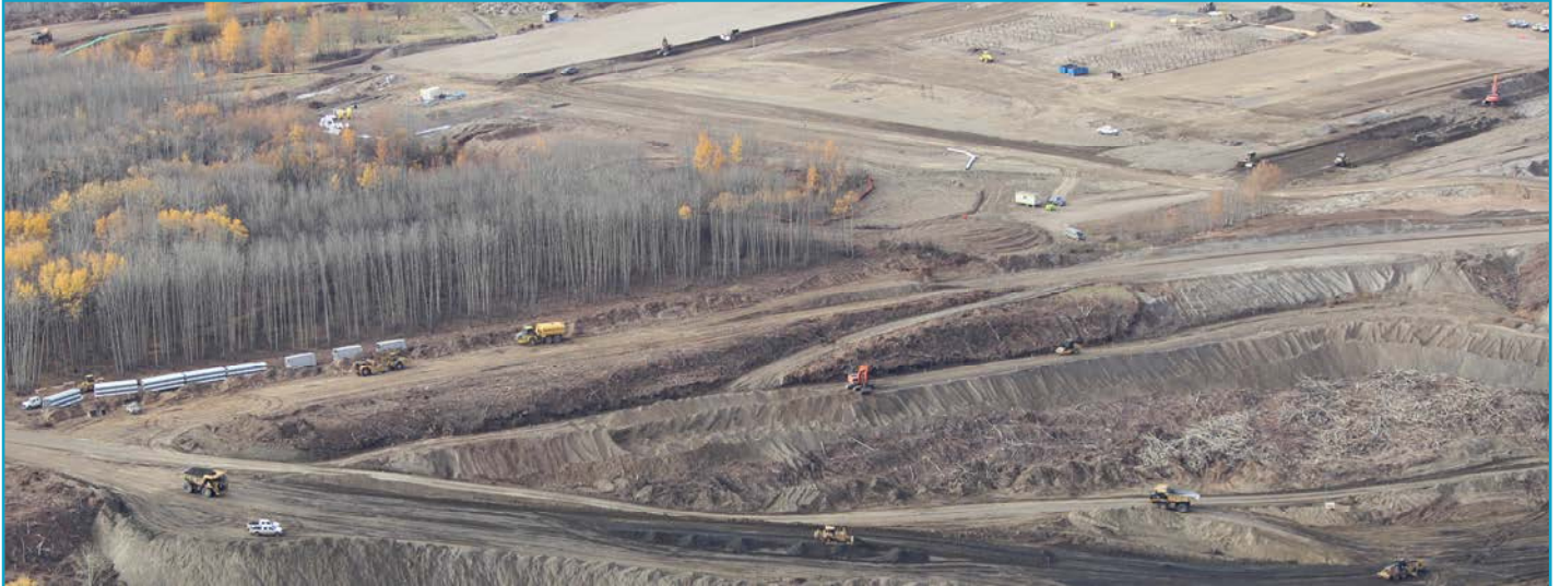
An aerial view shows material relocation at the Site C dam site.
