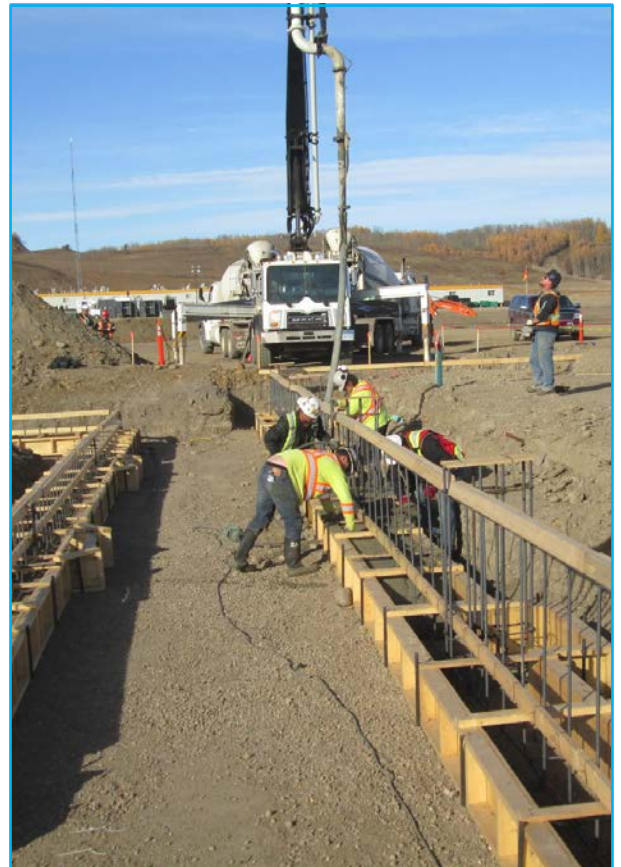
Workers from ATCO Two Rivers Lodging Group start the first concrete pour on what will be the worker accommodation fitness centre.
