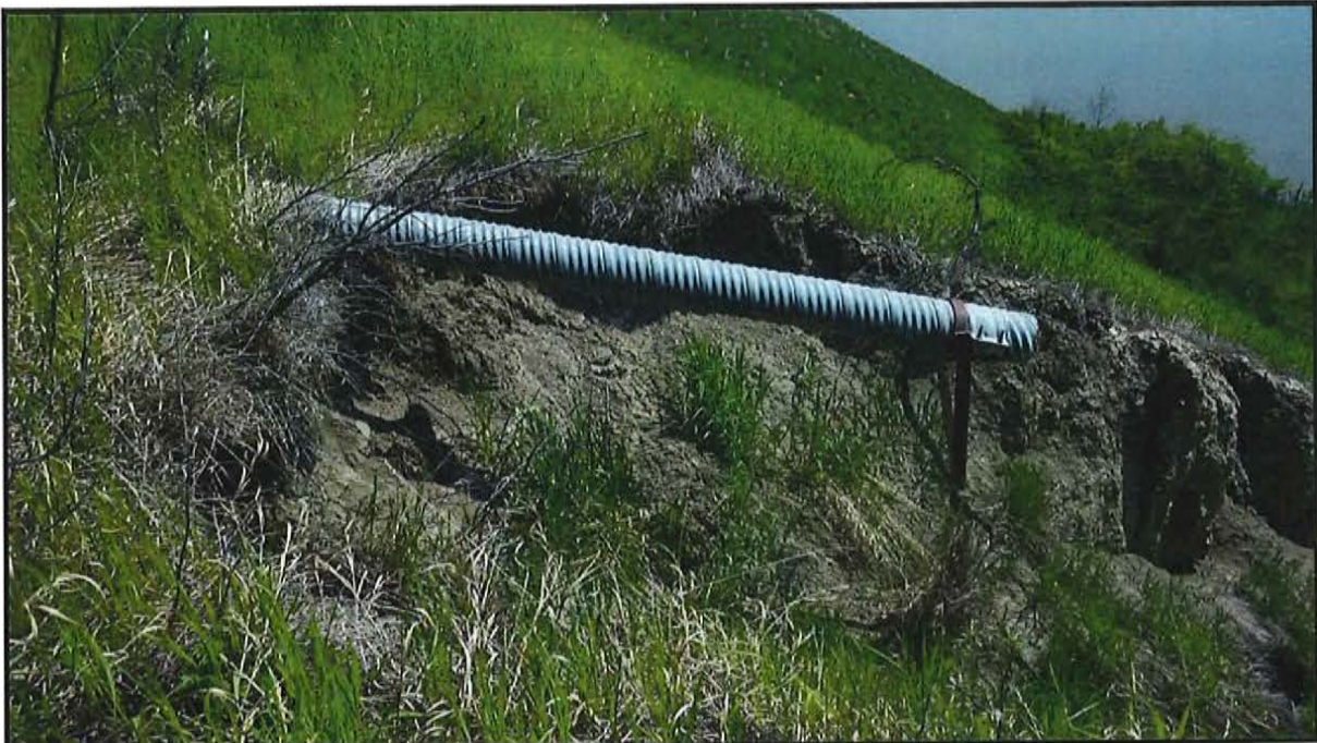
Photograph 2.1.2: Example of broken pipe and slope failure (Credit: Binnie)
