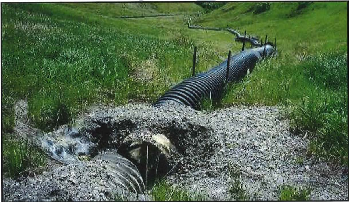
Photograph 2.6.1: Example of broken pipe (Credit: AMEC)
